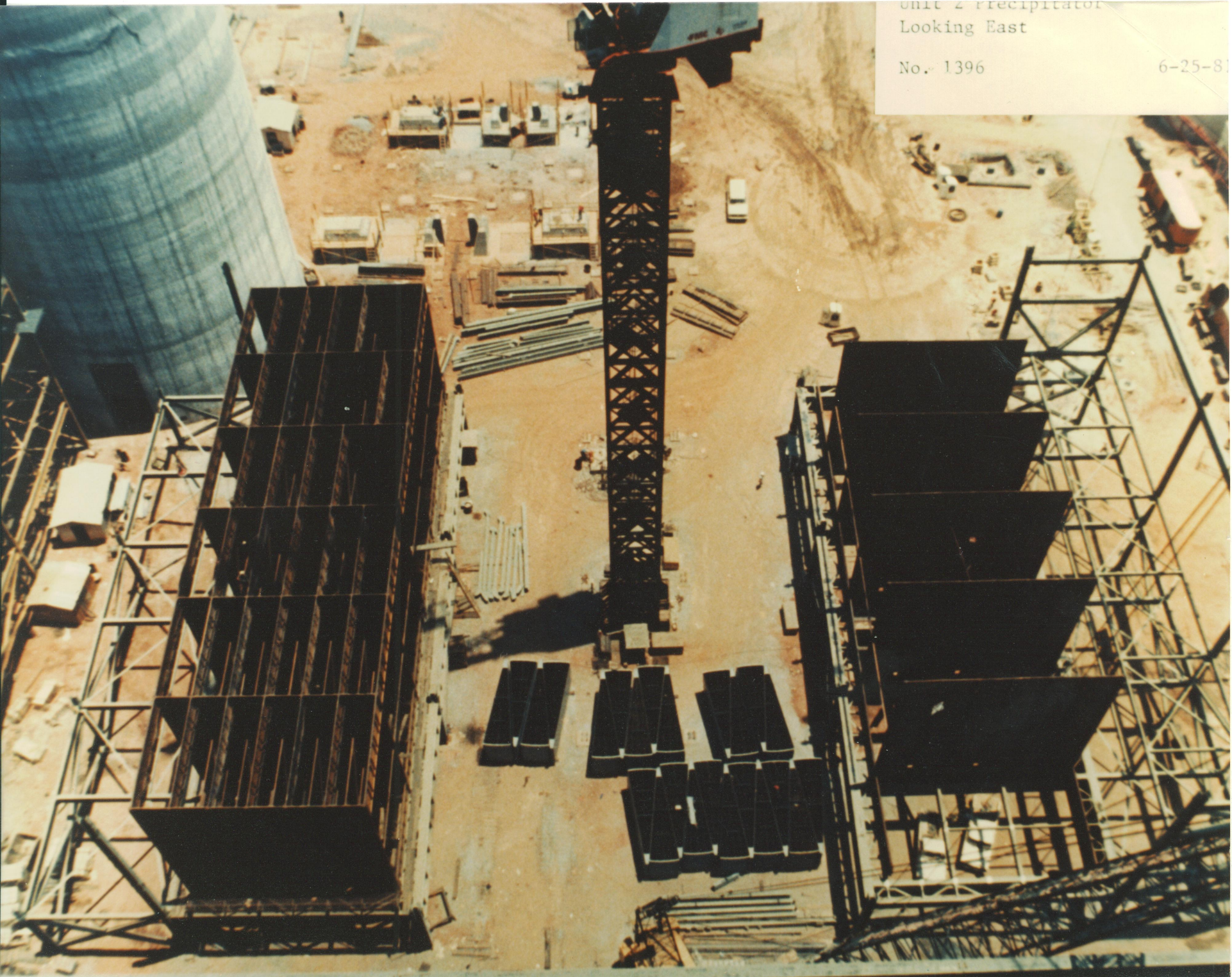
DELTA AIR LINES ATLANTA, GEORGIA BLAIR-BURDETTE, CONTRACTOR PATCHEN, MINGLEDORFF & ASSOC 1,975 TONS
